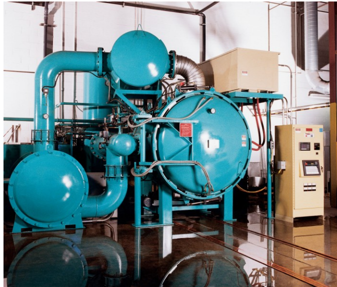
Representative medium-size furnace installation has a small floor-space requirement
